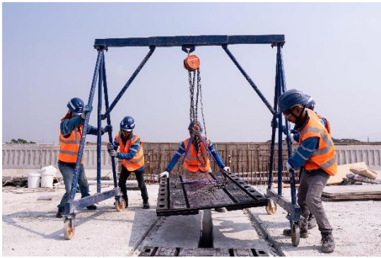
Installation of ISOSISM® SFX joints by specialized Freyssinet teams in Jakarta (Indonesia)
